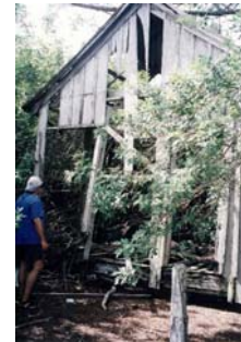
Site C-WCIND-2 - Abandoned structure at Rum Bay channel shoreline at the base of large Australian Pine
