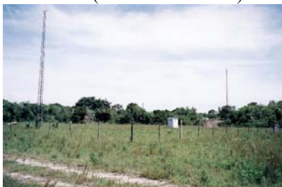
High voltage equipment area and antenna (southeast corner)
